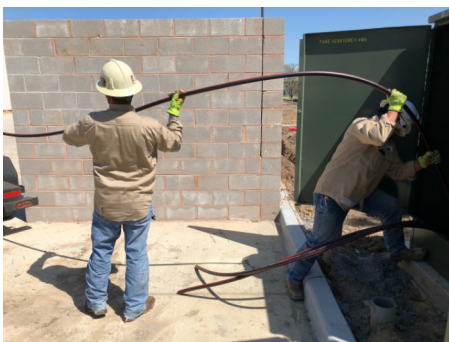
TNMP linemen put in new service for a commercial customer in League City, part of the growth continuing in the Gulf Coast region.
